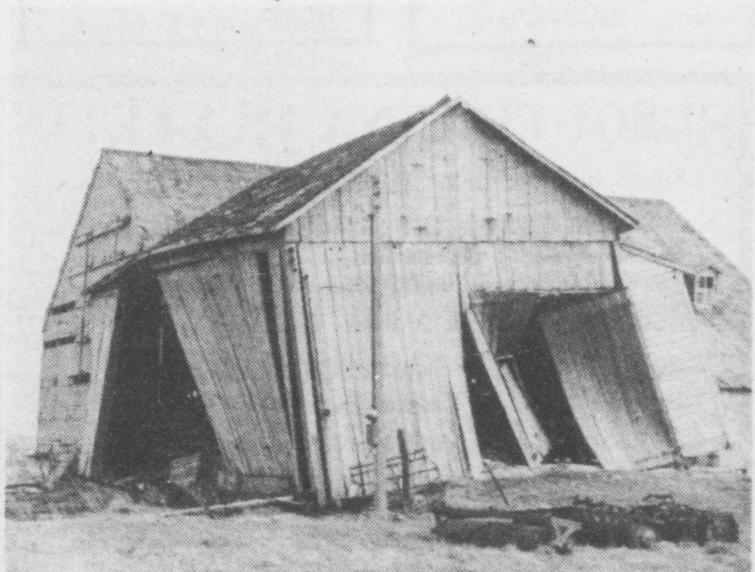
Damaged barn east of Maytown
