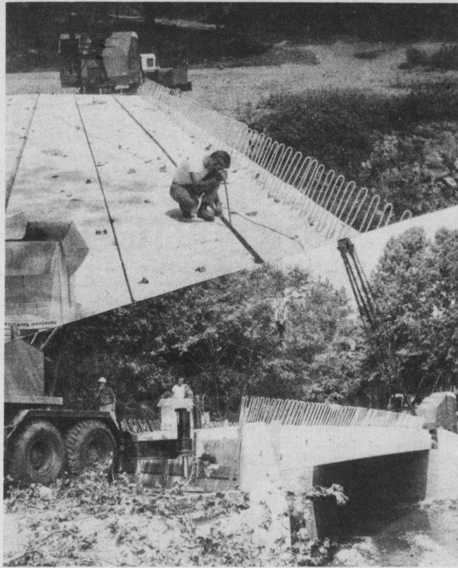
WORK IS PROGRESSING on the new concrete bridge over Little Chiques creek. The new structure replaces an old covered bridge swept away by the Agnes flood. It is located immediately north of Route 23 at the confluence of Big and Little Chiques.
