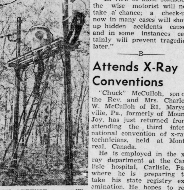
CIVIL DEFENSE siren at Winston-Salem, N. C., is installed by a fire department electrician on the Wake Forest College campus with the assistance and technical advice of Edmund P. Sullivan (on ladder), new city-county deputy CD director. Sullivan's salary is paid 50-50 by Federal and local governments as part of a nation-wide program to strengthen State and local civil defense units. (OCMD Photo)
