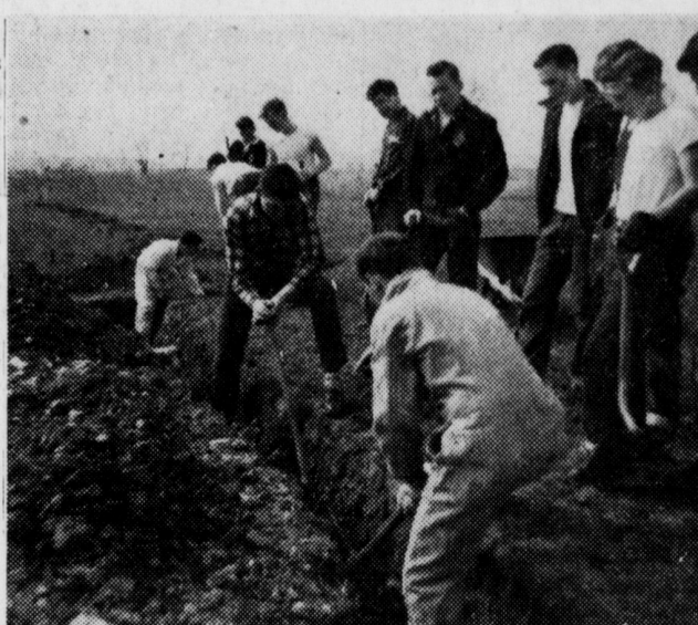
A school-service project, F. F. A. Members dig footings for the new Donegal baseball dugouts.
