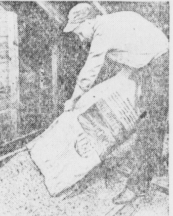
Zonolite vermiculite insulation being installed over ceiling of dairy barn at Mississippi Farms, Oregon, Ill.
