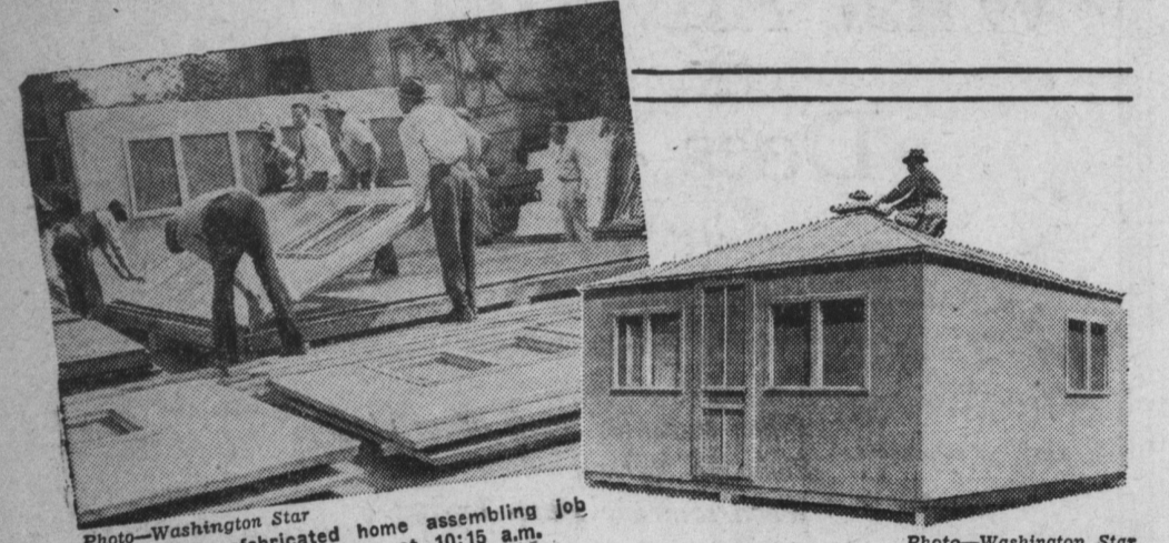
Photo—Washington Star Start of prefabricated home assembling job by inexperienced crew at 10:15 a.m. Photo—Washington Star At 11:10 a.m. the workmen had constructed the home, as shown above.
