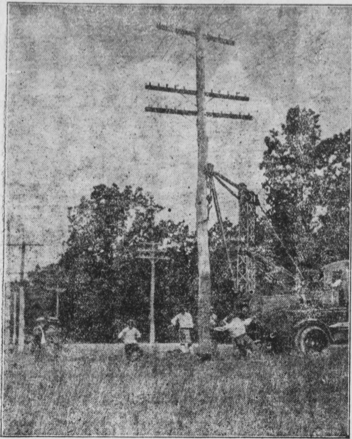
The post-hole digger which was the chief means employed in the moving of the pole line, consisting of one hundred and thirty poles and approximately fifty miles of wire. This device pulled the poles up out of the ground, dug the holes at the new locations and placed the poles.
