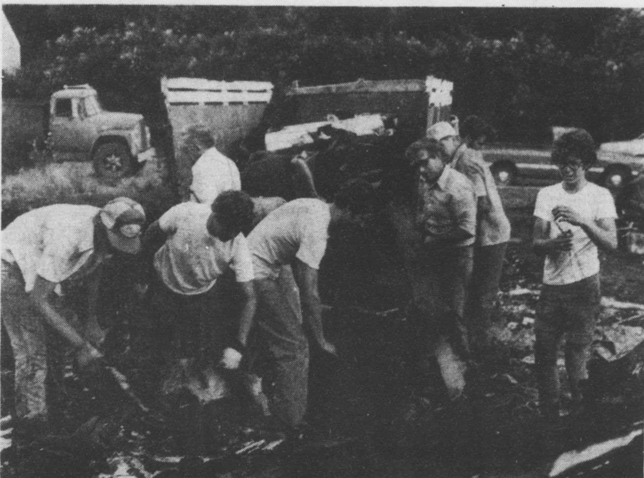
Volunteers of the Mennonite Disaster Service are shown at work in Marietta. The burned-down house they are working on is north of Gay Street on Walnut. The MDS has 2600 members in the U.S. and Canada. They don't charge for their services. The MDS volunteers plan to finish the job this Thursday evening.
