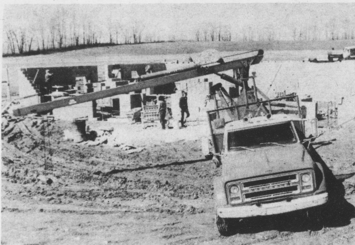
Construction is proceeding on the new Maytown-Marietta medical center on Route 441. The center will be affiliated with St. Joseph's Hospital in Lancaster.
