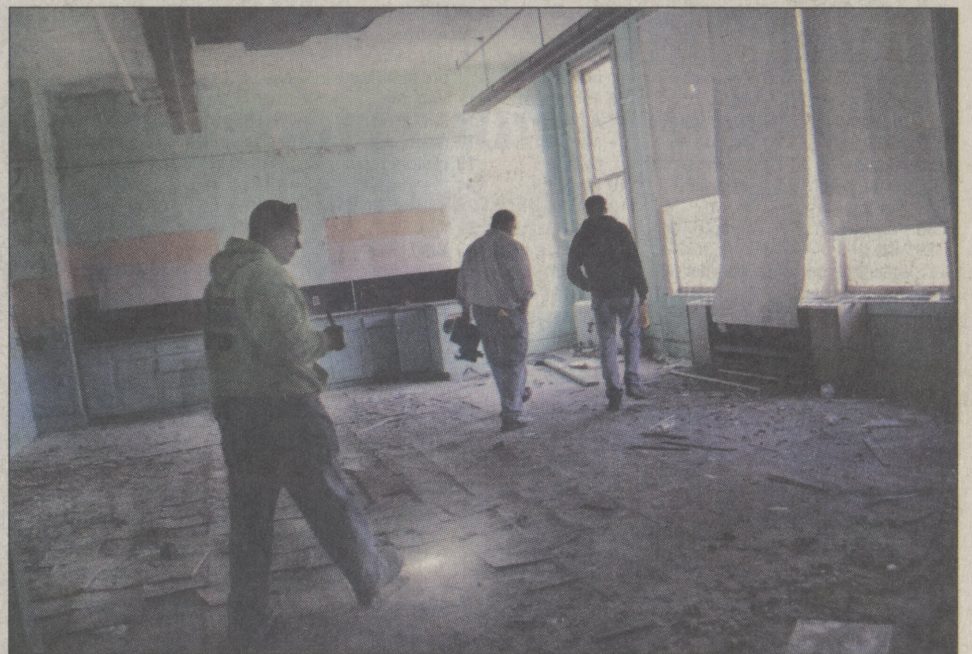
Charlotte Bartizek | FOR THE DALLAS POST About 20 companies walked through the old Dallas Twp. High School building with hopes of winning a bid for its demolition on Wednesday, Oct. 30. Mark Kraynack and Nick Dennis from the Dallas School District, right, show one of the representatives around the building, which was built in 1927.
