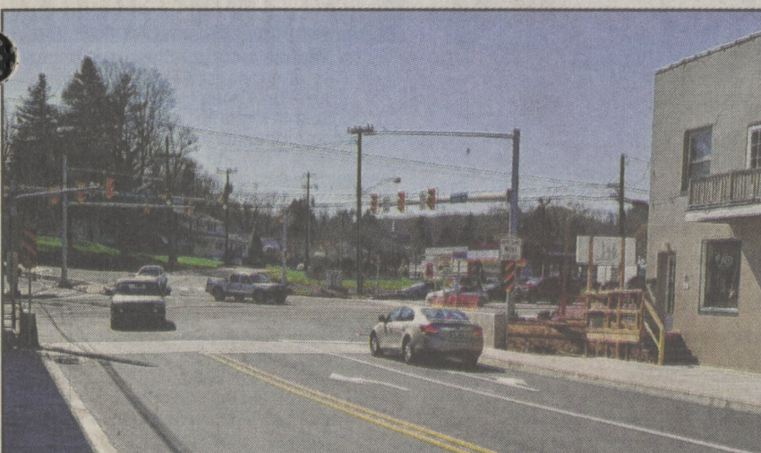
The bridge on Center Street in Shavertown opened April 21 after being closed for repairs for nearly a year.
