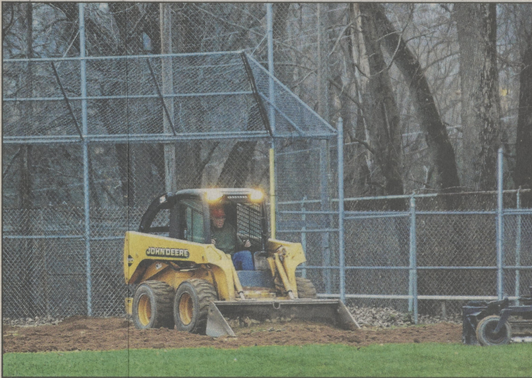
Crews work well into the night to put new dirt on the upper fields.
