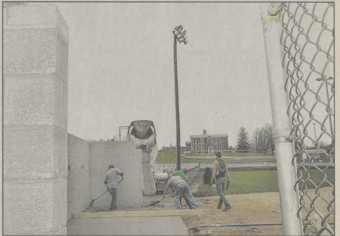
Richard Hiedacavage, of Harding, and his construction crew pour concrete and assemble new dugouts at Kubis Field in Dallas.
