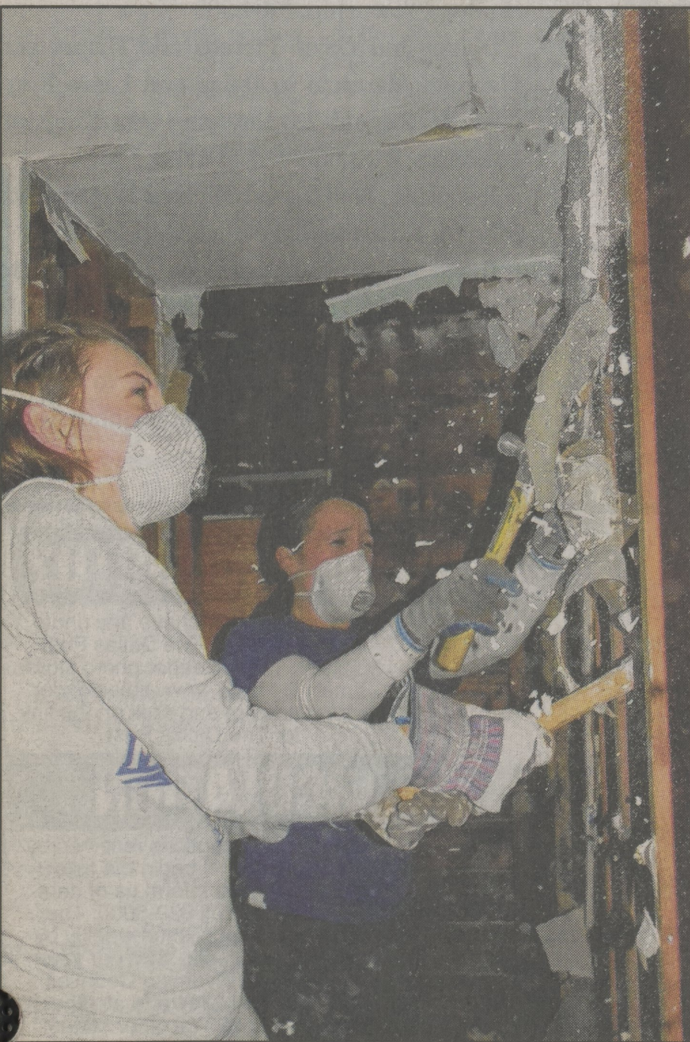
Misericordia University students Caroline Landen, left, and Kellyann Gough rip water-soaked drywall out of a home on Staten Island.
