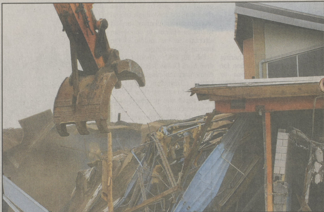
Workmen carry away asbestos material while bricks from the old Dallas High School would be crushed and recycled as the foundation for the new parking lot in June.
