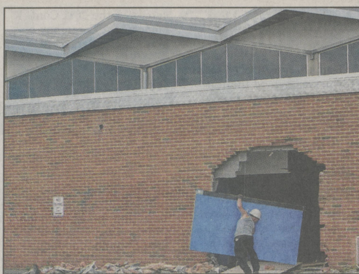
Charlotte Bartizek Photos/For the Dallas Post Workmen carry away asbestos material while bricks from the old Dallas High School will be crushed and recycled as the foundation for the new parking lot.
