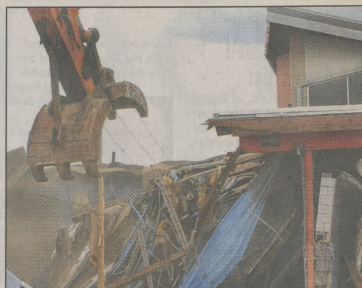
Demolition work continues on the old Dallas High School building to make way for the new one.
