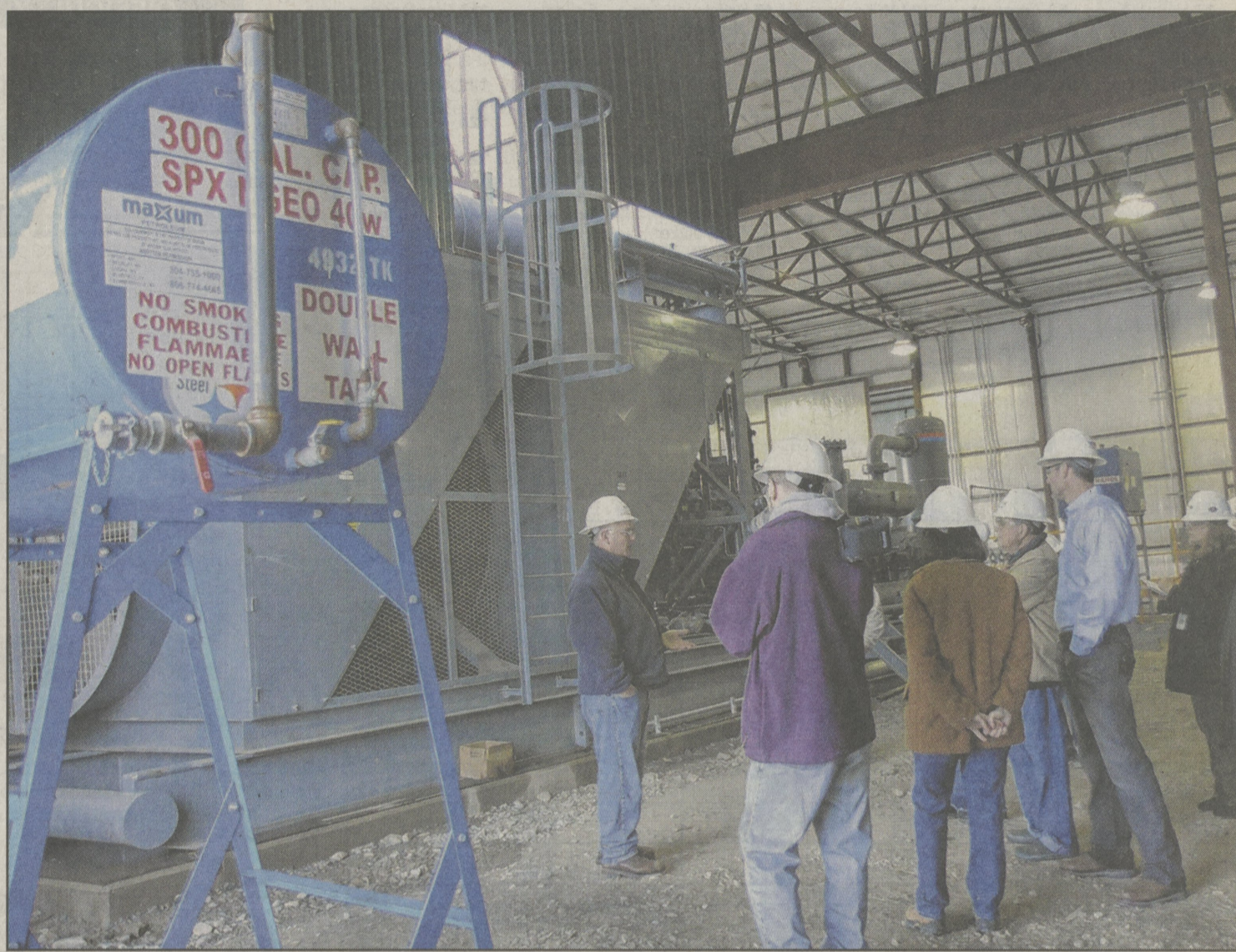
Operations manager Steve Hamilton explains the inner workings of a newly-erected c3 unit compressor station on a five-acre site in Hop Bottom.
