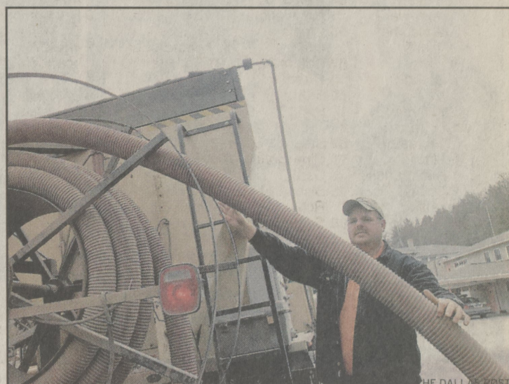
Jay Wilkes helps guide tubing for environmentally-friendly fill toward a new piece of property next to the town hall. The additional area will help with the town's recent recycling problems.
