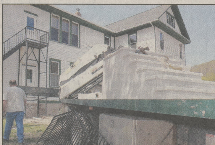
Workers from the Scranton Concrete Step Units place modular stairs under the door to the Schenk Library in the Old Noxen School building. A time capsule was also placed under the stairs.
