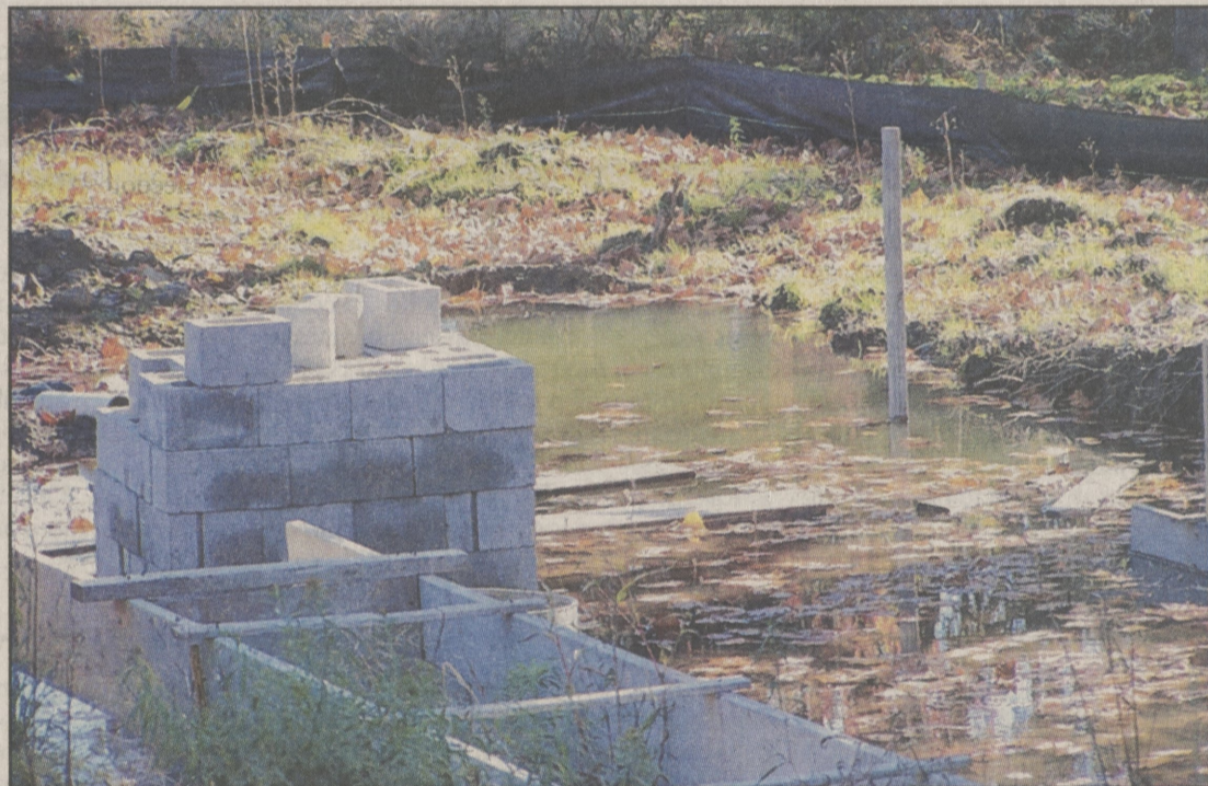
Rainwater fills a hole at a construction site on East Fallbrook Avenue in Dallas Township. The project was abandoned after the township pulled the developer's building permit because of a void subdivision and drainage issues. Neighbors are worried children will get hurt.
