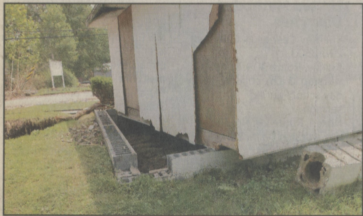
The Sportsman's Club of Noxen was pushed from its foundation during last week's flooding.
