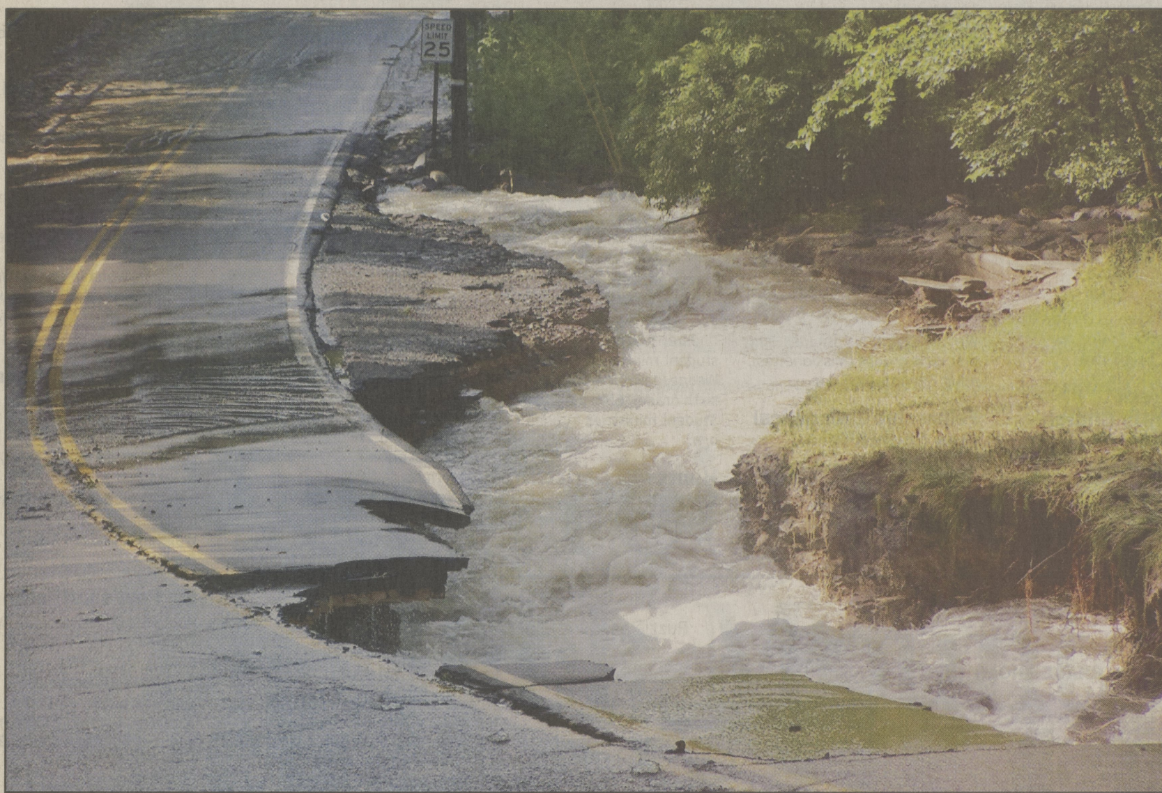
A section of Hillside Road near the five-way intersection at the Huntsville Reservoir was completely destroyed.
