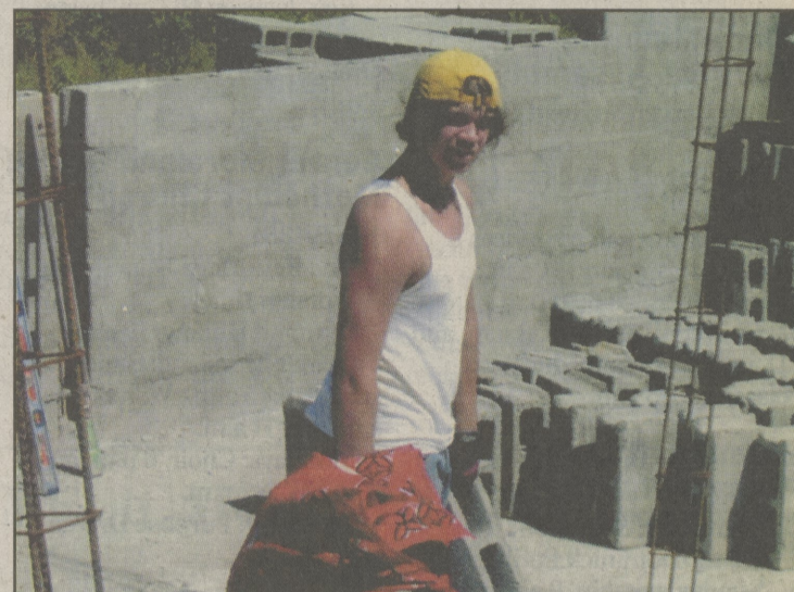
Dallas High School student Mark Evans carries a few cinder blocks while helping to build a small health clinic in Honduras.
