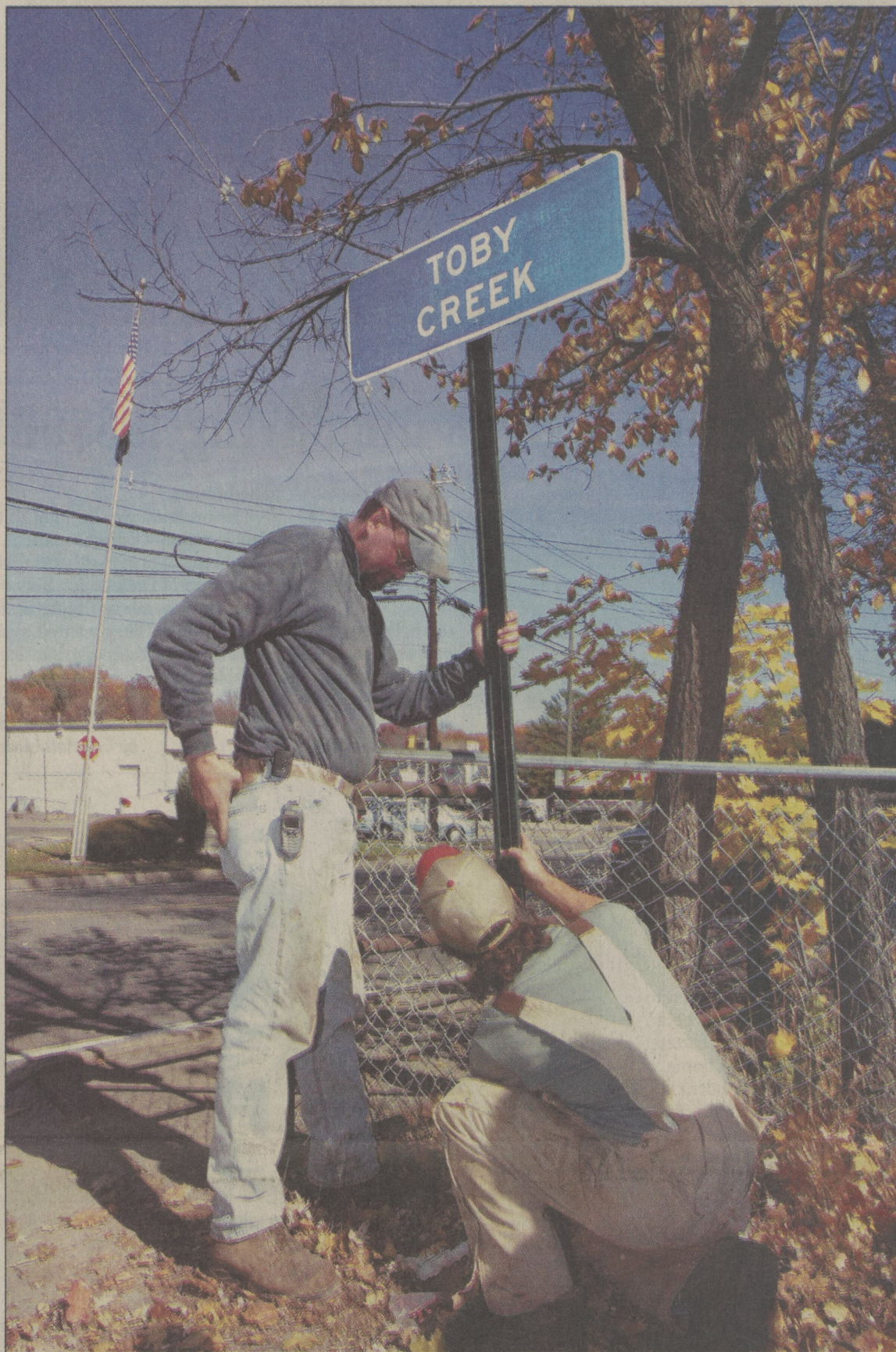
John Cybulski and Frank Kus, Dallas Borough maintenance workers, install the first of 12 signs that identify where Toby Creek crosses under a roadway. This one is at the corner of Machell Avenue and Route 415.
