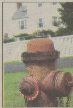
Fire hydrants like this one in Cedar Lane will be usable once the water company installs a storage tank
