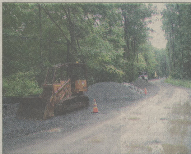
With skies threatening, construction equipment sat idle June 22 along Green Road in Kingston Township.
