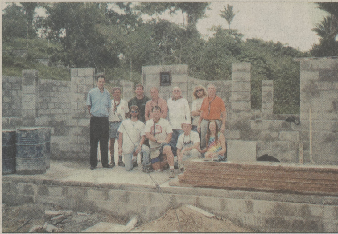
On their last trip to Honduras, volunteers began construction on a new school.
