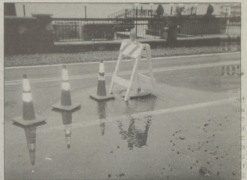
Water pressure from a sanitary sewer line forced the top of a manhole cover out of place. As a result raw sewage poured out, eventually making its way to a grate and directly into the lake. The Department of Environmental Protection (DEP) said the problem could mean the borough is in violation of The Federal Clean Water and Streams Act. An investigation is pending.
