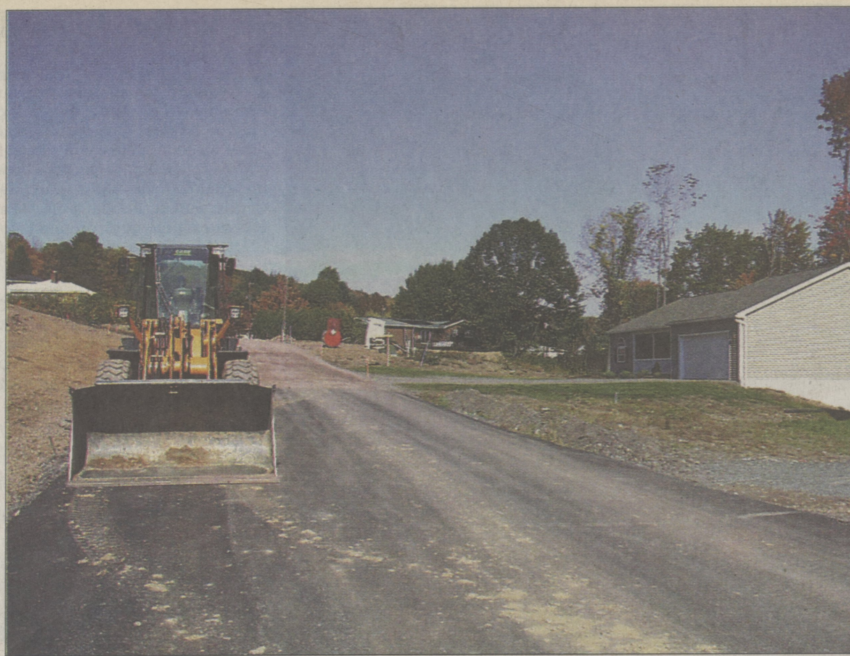
Lehman Township Supervisors say drainage and roadway issues in The Pines development haven't been addressed.
