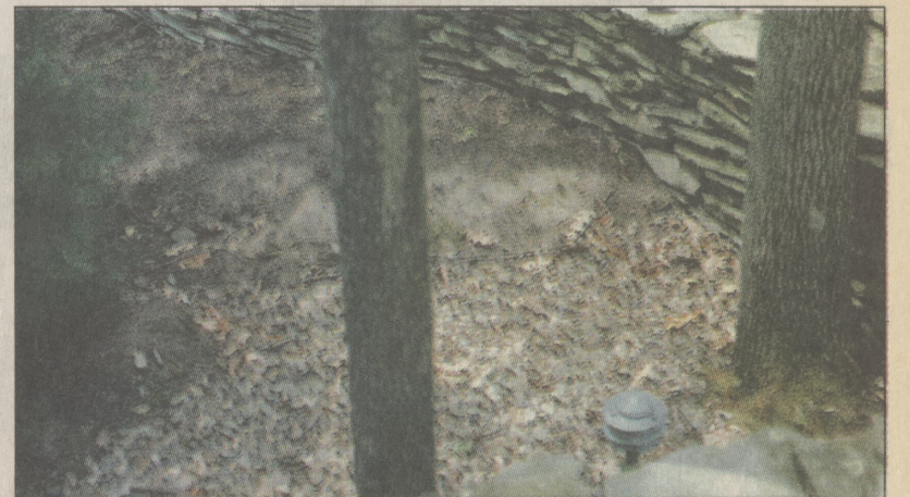
Water runs from an adjoining property under the stone wall that borders David Kolesar's land.
