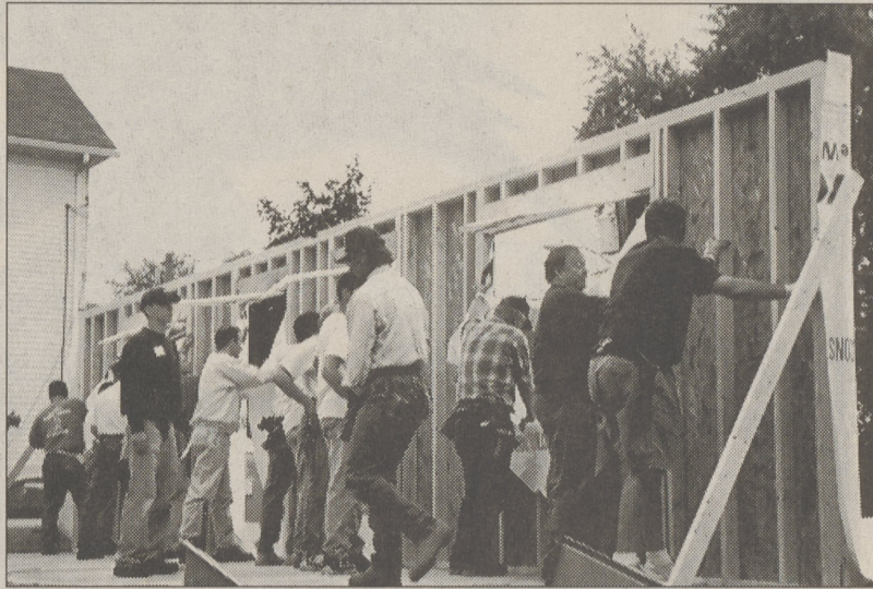
Habitat for Humanity volunteers from Trinity Presbyterian Church put up one wall of a home in Wilkes-Barre
