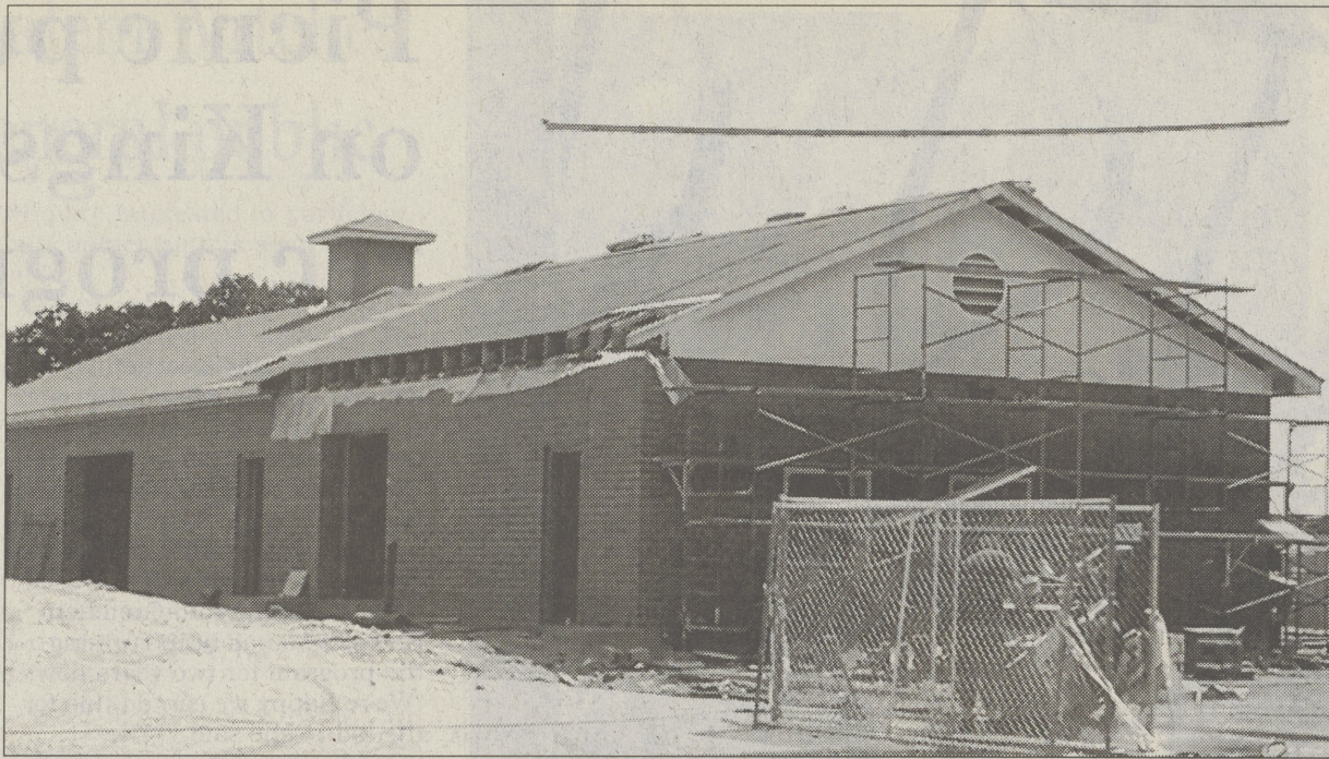
POST PHOTO/BILL GOODMAN The concession stand at the Dallas High School football field is almost ready for business. Workers have put the brick facing on the walls and the inside is nearly finished.
