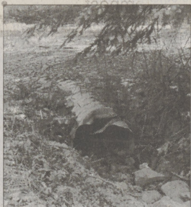
Hemlock Gardens storm drains send sediment to Harveys Lake.
