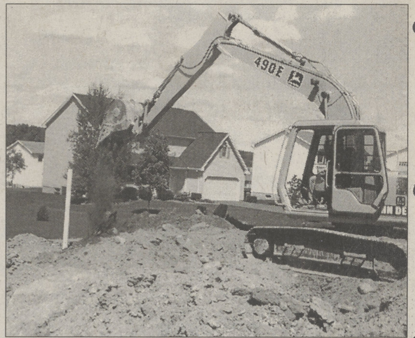
Ernie Slocum, Lehman, working for Lehman Homes, dug the cellar for a new home in Meadowcrest, Jackson Twp.
