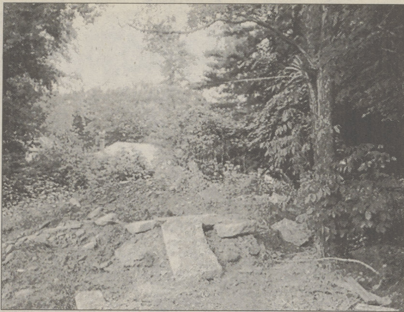
Waste material is piled along the roadside in the Oak Hill development, as National Utilities has begun but not finished a water main replacement.
