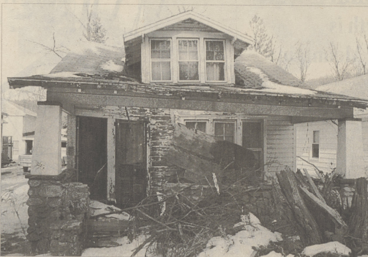
This abandoned house on Old Lake Rd. is one of many the Borough of Harveys Lake would like to tear down. The borough has applied for a county demolition grant of $15,000.
