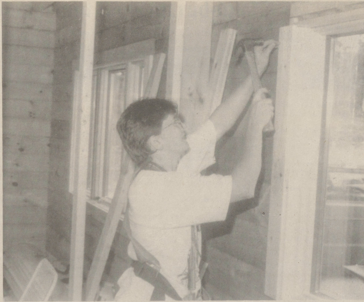
Finish carpenter Wendy Flick of Chestnut Ridge Construction applies moulding around a thermal window at the Luzerne County Conservation District's new log office building in Jackson Township.
