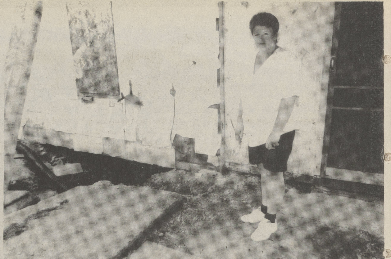
Betty West stands by her back porch, which she had to remove to find a water leak which also damaged part of the foundation of her home on Second Street at Harveys Lake.
