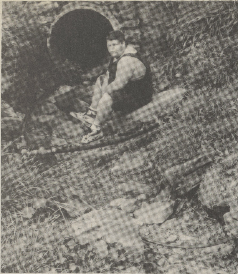
Charles West shows where exposed water lines follow a creek bed and run through a culvert at Second Street at Harveys Lake.
