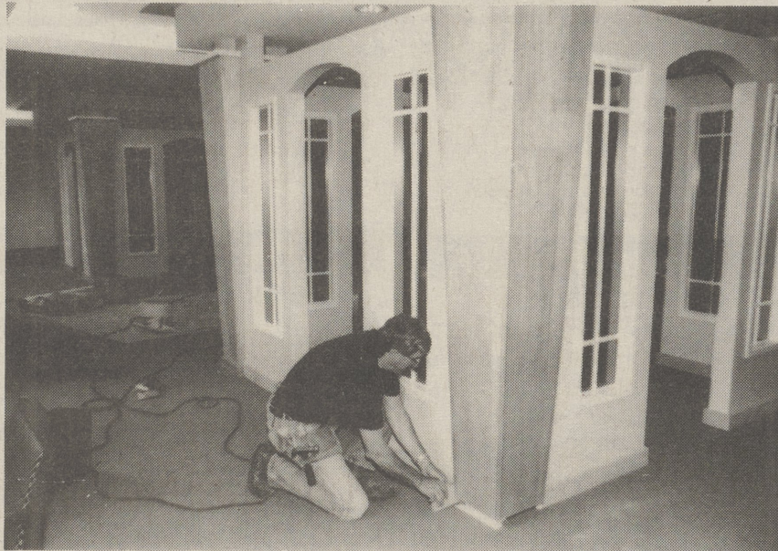
POST PHOTOS/RON BARTIZEK Larry Randall, above, of Sordoni Construction Services, attached baseboard to a waiting area in the new Dallas Family Practice building. The entrance is shown at right. There will be an open house Saturday at the facility.
