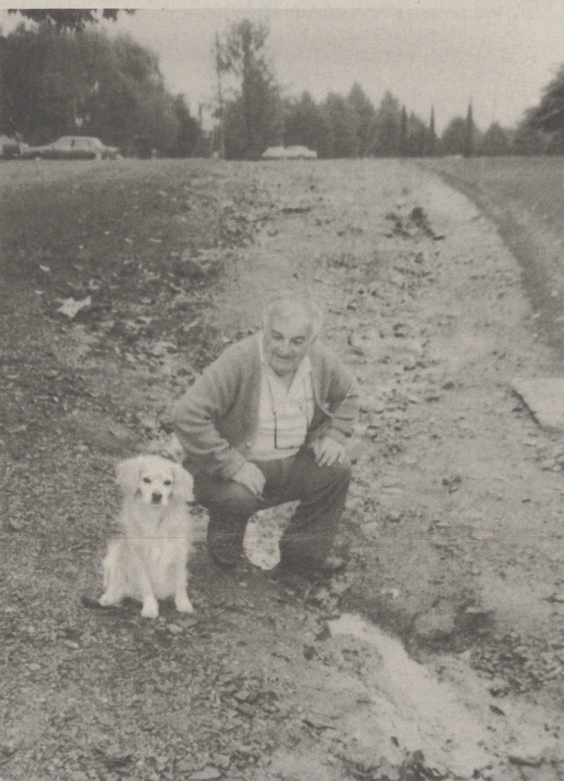
PROBLEM ROAD - Crown Hill Village resident Walter Baseski and his friend, Lady, show one of the many deep gullies in the development's three roads.
