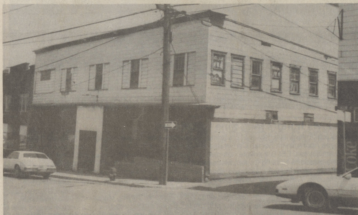
COMING DOWN SOON - The former Hearthstone Pub building in the center of Dallas Borough may finally be torn down if the borough receives a state grant it has applied for. The building is so dilapidated that the Dallas Fire Company is under orders not to enter it should it burn. (Post photo/Grace R. Dove)
