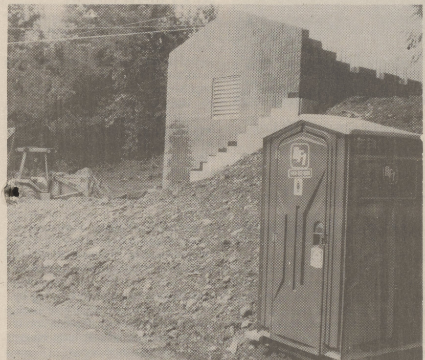
POINT OF CONTENTION — Work continues on this pump house on Old Route 29 near Mizdail Road in Jackson Twp. despite repeated warnings that it violates township setback ordinances.
