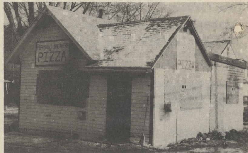
FIRE DAMAGE - Pepperoni Brothers Pizza on Franklin Street, Shavertown, was heavily damaged in a fire early Thursday morning, March 12. (Post photo/Grace R. Dove)
