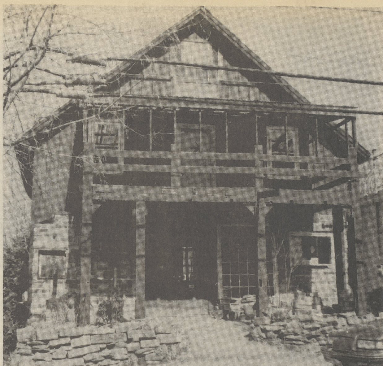
REFURBISHED - A 120-year-old barn at 66 Main St., Dallas, has been divided into an upstairs apartment and a downstairs storefront during extensive renovations by its new owner, Scott Parkhurst. (Post photo/Grace R. Dove)
