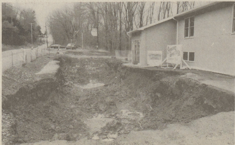
TAINTED SOIL SITE - The parking lot at Jackson Township's new municipal building is now a crater after old gas tanks were removed from ground in front of the former gas station. The old tanks tainted the soil around them with gasoline. (Post Photo/Eric Foster)
