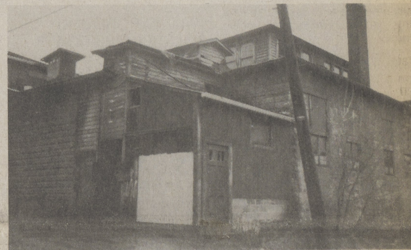
EYESORE AND DANGER - The former Hearthstone Pub on Main Street in Dallas is regarded as dangerous by local fire and police officials. (Post photo/Grace R. Dove)
