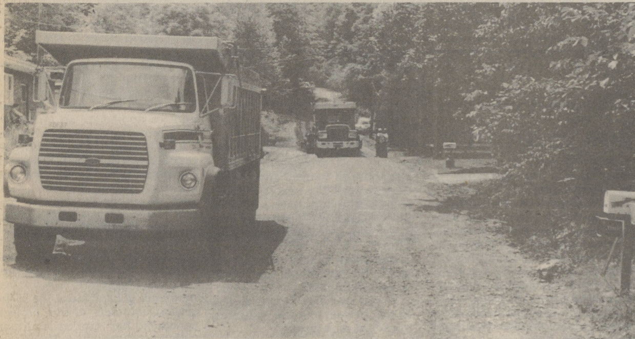
ROAD REPAIRS - The "tar and chip" program is underway at Harveys Lake. This section of road at Keefer Plot is the first of many roads to be resurfaced this summer as part of the project. (Photo by Scott A. Davis)
