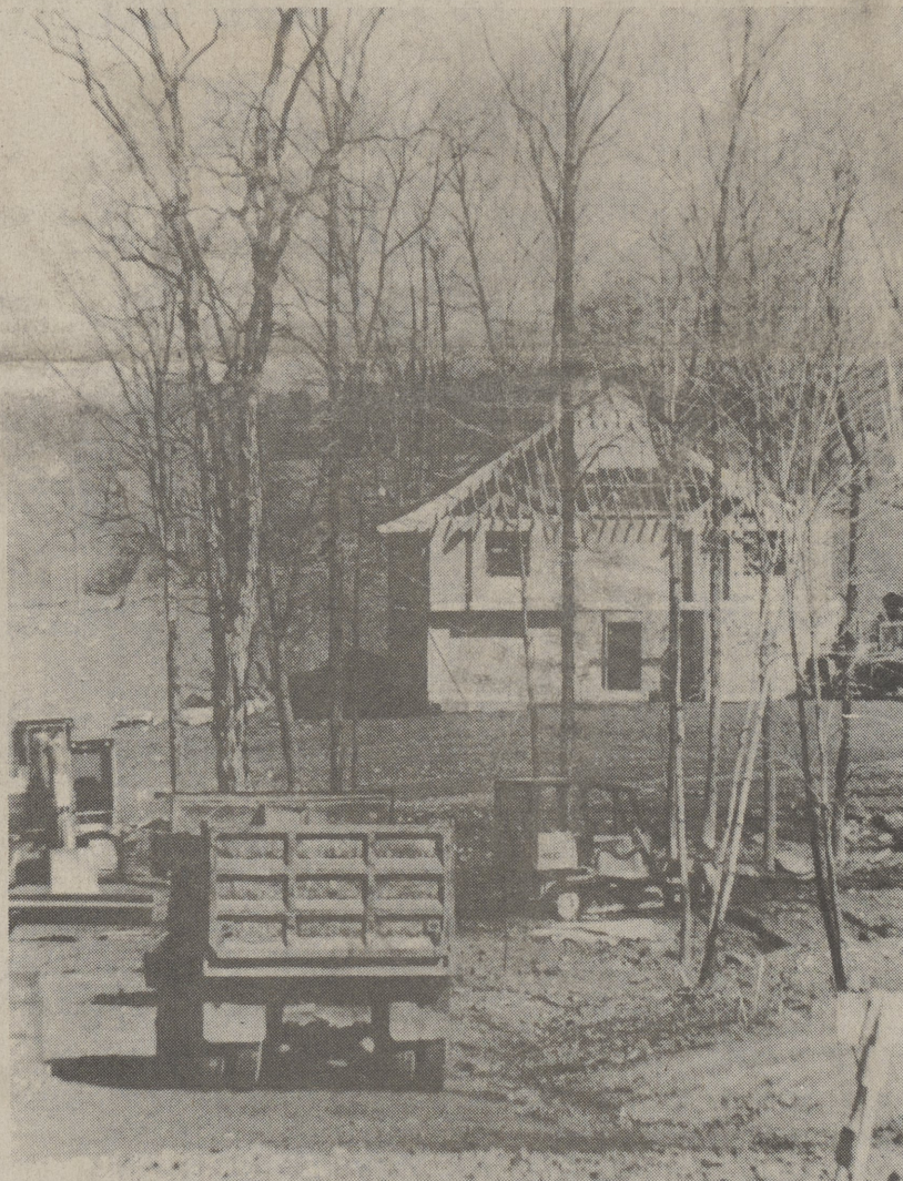
VIOLATIONS TO STOP - A new home was under construction Monday in Phase II of Sunrise Estates, off Carverton Road in Trucksville. The developer has been ordered to stop work on portions of the project that are in violation of Kingston Township ordinances. (Photo by Ron Bartizek)
