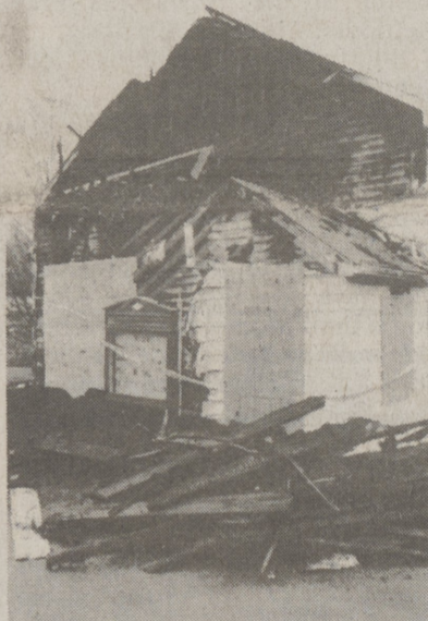
ARSONIST'S WORK - The Beaumont Union Gospel Church building sustained heavy damage to its vestibule in a fire last week. (Photo by Ron Bartizek)
