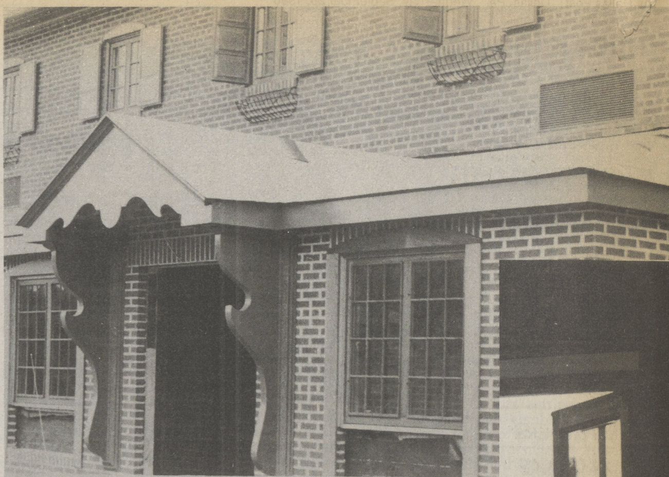
BEAUMONT INN Contractors are busy renovating Beaumont Inn to be ready in time for the Thanksgiving Holiday. Above is the front of the building being remodeled similar to the Inn in 1948. At right is a view of the Tunkhannock Hills from a newly remodeled guest room window. (Charlotte Barizek photo)
