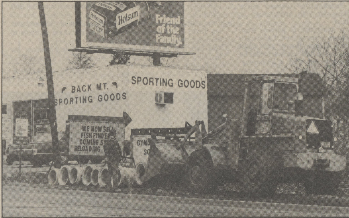
GET READY FOR MORE JAMS! — Penn DOT crews begin assembling equipment and materials for construction work to be done on Rt. 309. The work is scheduled to begin on March 31, and it will continue until September. (Linda Shurmaitis Photo)
